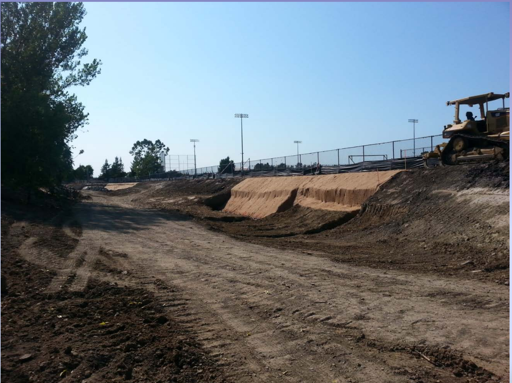
A blanket made of natural fibers covers the bare soil, to reduce erosion.
