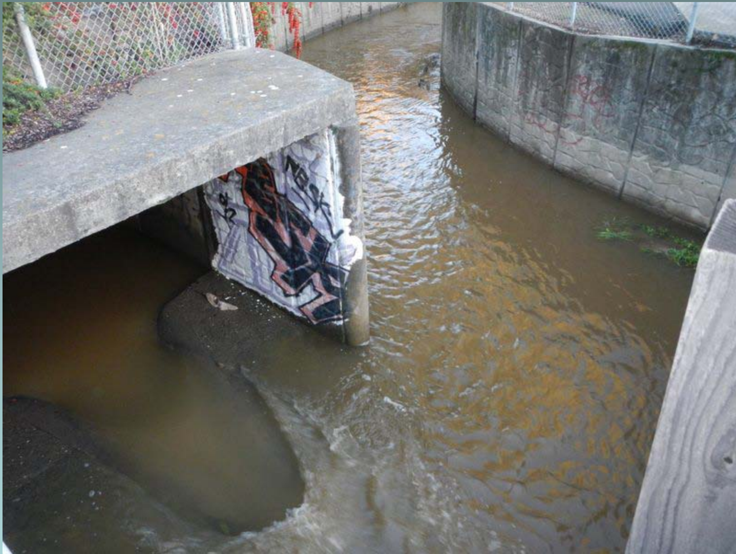
The Colgan Creek Box Culvert, where Kawana Springs joins the water coming through the underground pipe from the neighborhoods around the fairgrounds and Colgan Avenue.
